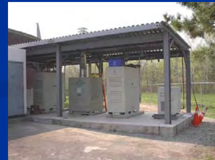
Lewiston Wastewater Treatment Plant
