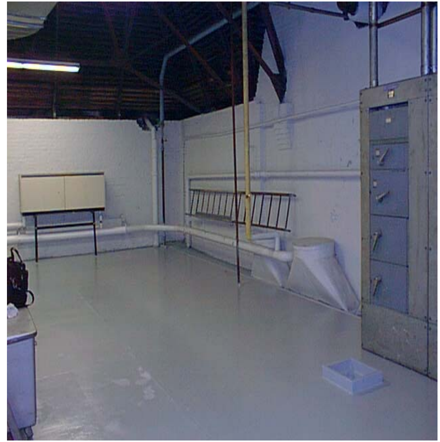
Cooling Tower Room - After
