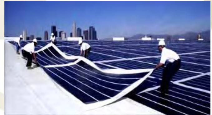
Building- integrated thin-film PV
